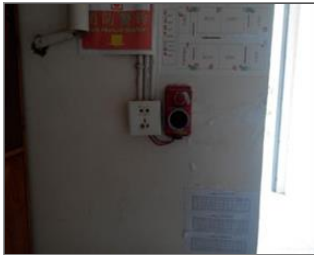
Photo of fire safety equipment Fire alarm.jpg
