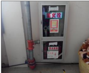
Photo of fire safety equipment Extinguisher and fire hydrant.jpg
