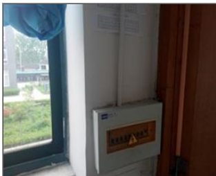
Photo of fire safety equipment Electrical box.jpg
